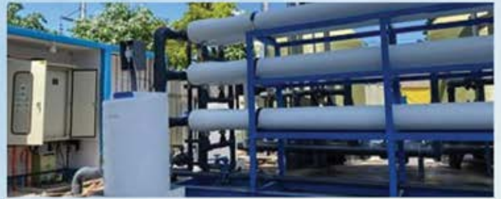
Energization of Victoria, Laguna Facility (Mar 2020)
